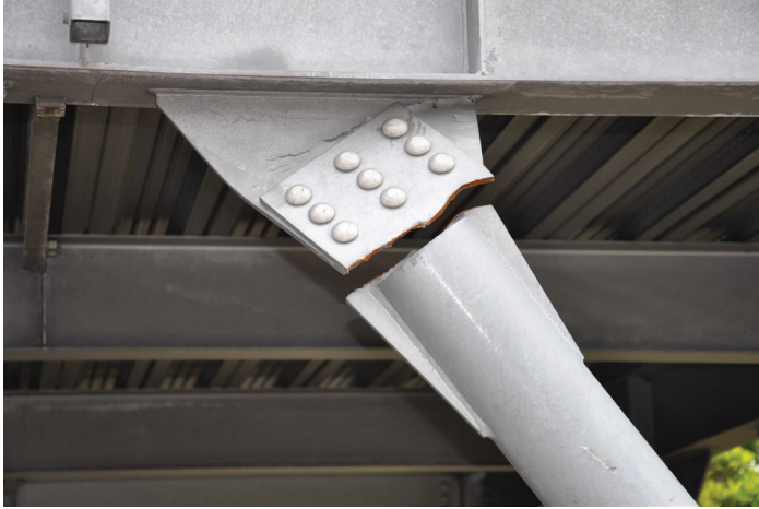
Figure 1.1. Effects of the 2011 Tohoku Japan Earthquake. Fracture of top gusset plate in the 2-story parking garage [165]
