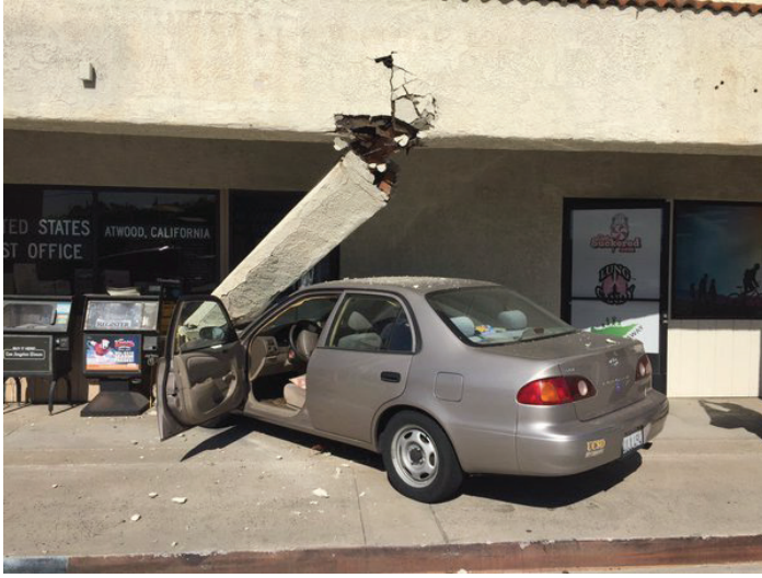
Figure 1.2. Structural failure after car crash into column in Placentia, California [142]
